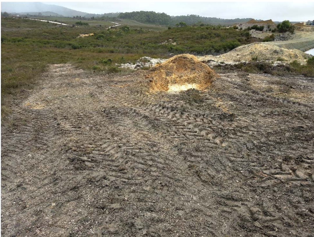
Figure 1 – Commencement of construction of the new Tailings Storage Facility at Granville Tin Project
